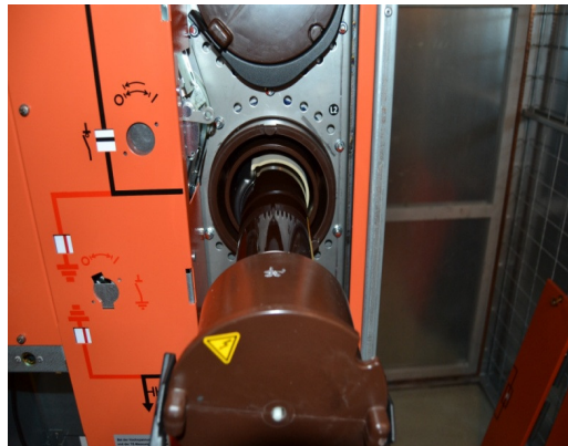
Fuse with switchgear
